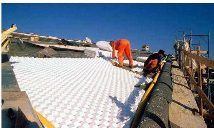
Installation of the drainage element Floraset® FS 75 on the pitched green roof area.
